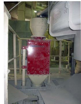
Production control for screening machine.
