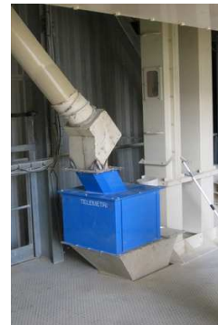
Loading control of silo for wheat flour.
