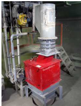
Loading control for bulk cement trunk under silo
